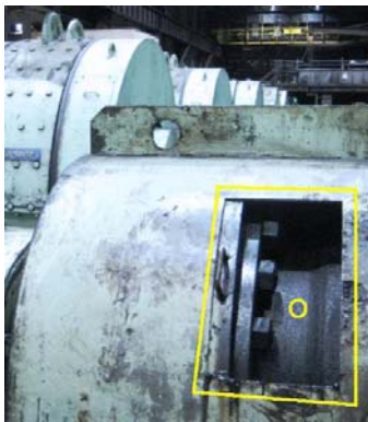
High vibration readings discovered in main gearbox.
